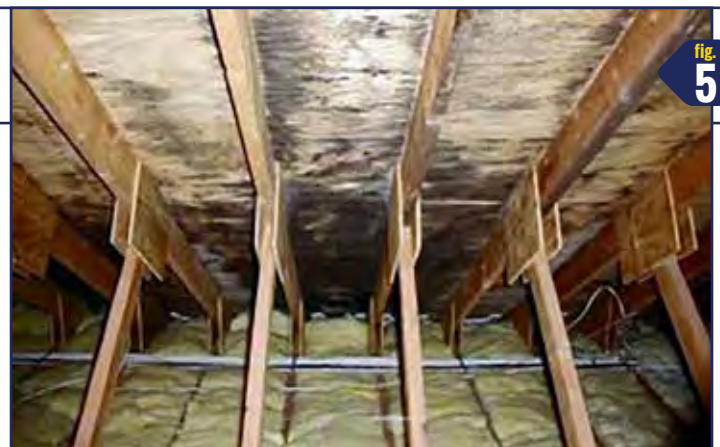
Moisture problems can often lead to mold issues, as shown in this attic.
